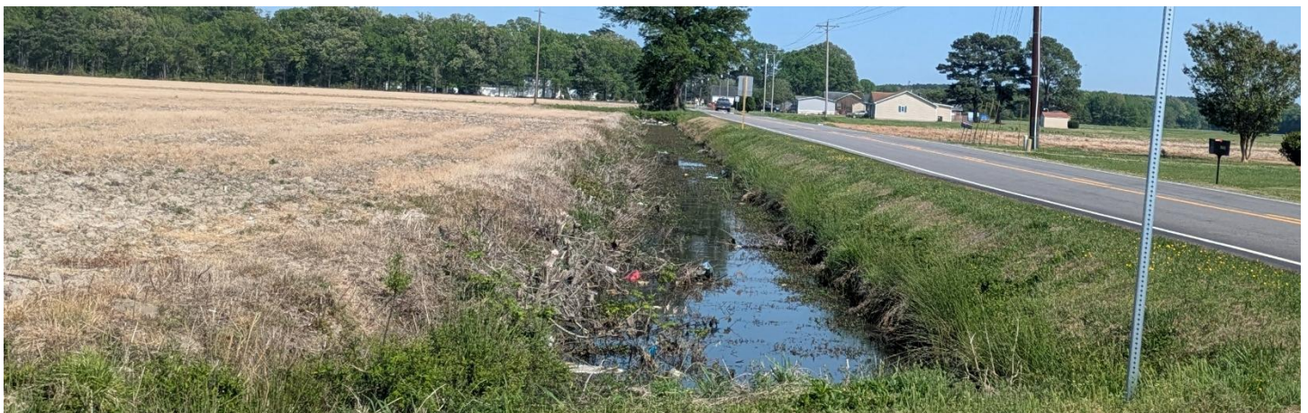
Figure 16. Drainage channel, Weston & Sampson
