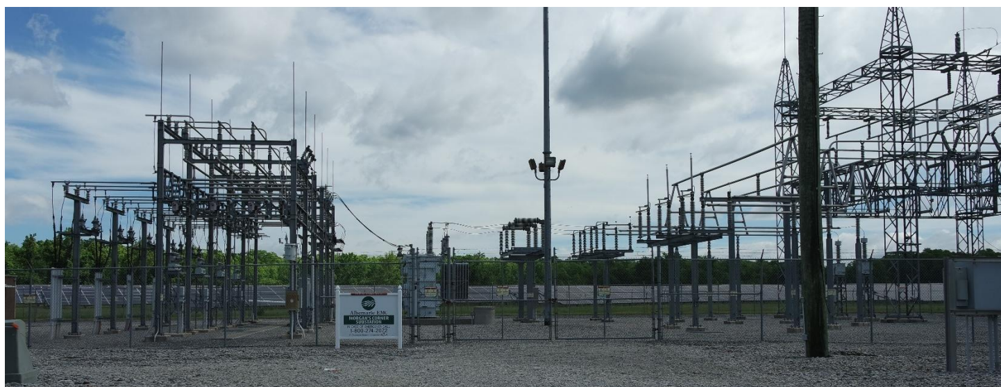
Photo 8. Pasquotank County Substation, Weston & Sampson
